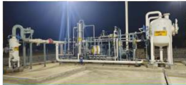
Vapour Recovery Unit for Truck Loading Facilities, RIL Rewari, Haryana
