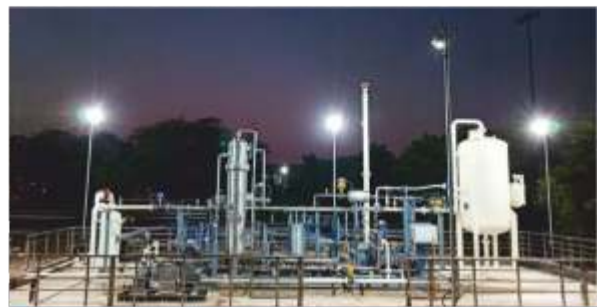
Vapour Recovery Unit for Truck Loading Facilities, BPCL Bharatpur, Rajasthan
